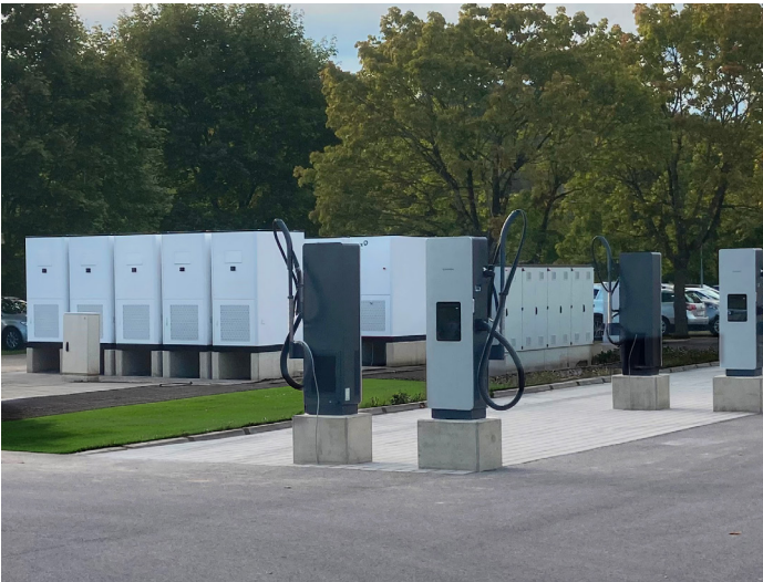
EV CHARGING PLAZA WITH CO-LOCATED G-MAX STORAGE
